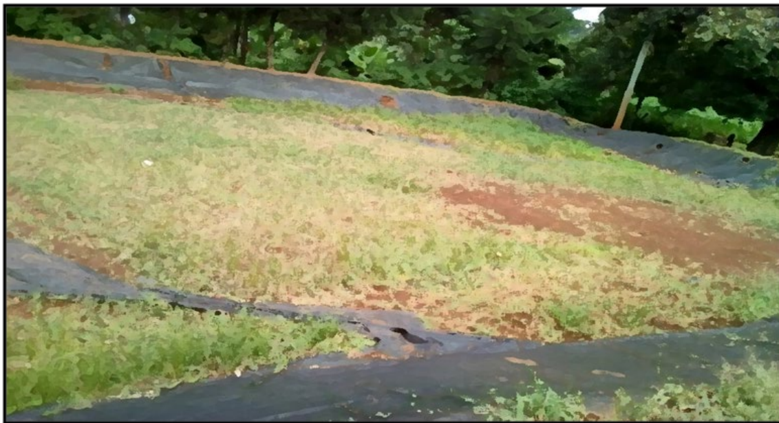
Figure 3: Pond within Kogony, Central Kisumu Ward not fully Covered by a Pond liner
