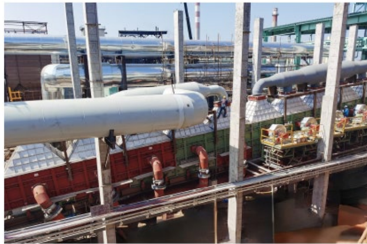
Figure 6: Operation Picture of the Super Steel Belt Dryer System at Phase II solid Waste Disposal Center Project in Baosteel Zhanjiang Iron & Steel Co., Ltd
