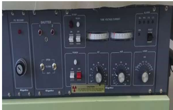
Figure 5: External Control Panel
