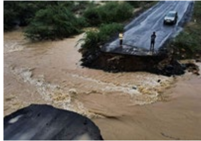
Figure 13: Broken Bridge, After Cyclone Biparjoy Made Landfall, Along the Naliya-Bhuj Highway
