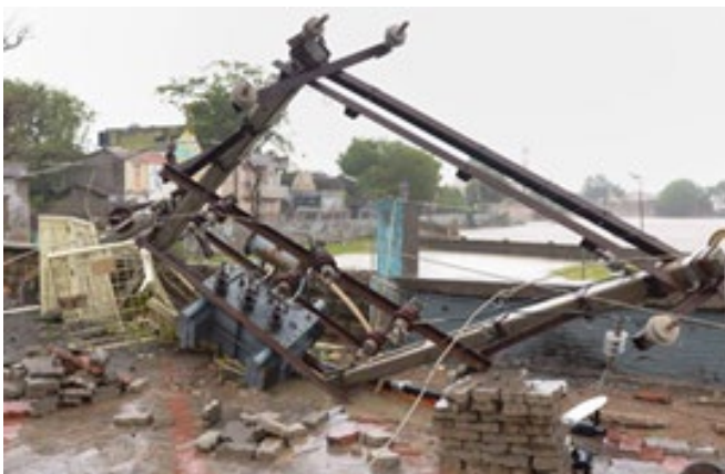
Figure 15: Electric Transformer Damaged at Mandavi on 16th June, After Landfall of Cyclone Biparjoy. (Photo: - Sam Panthaky/ Afp Via Getty Images)
