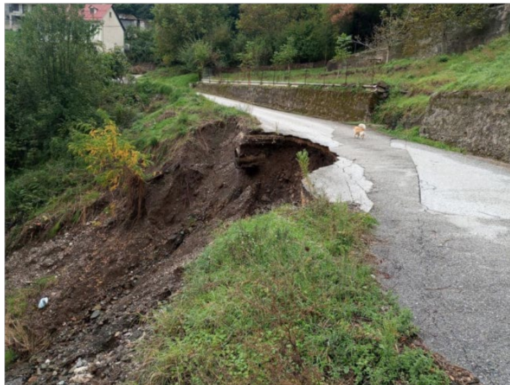
Figure 7: Road Damaged by Landslide After Heavy Rainstorm
