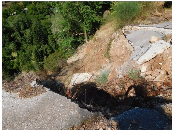
Figure 2: Road Collapse on Steep Ground
